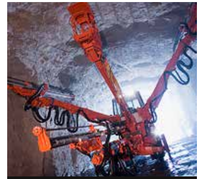
Two Sandvik DT1131i and two DT921i will excavate the world's longest subsea tunnel.
